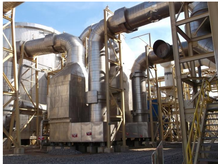
Sulfuric Acid Plant Ducting
