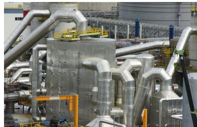
Ducting Around a Converter
