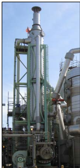
NORAM Preheat Heat Exchanger
