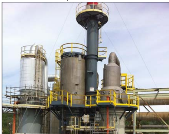
NORAM Dry and Final Acid Towers
