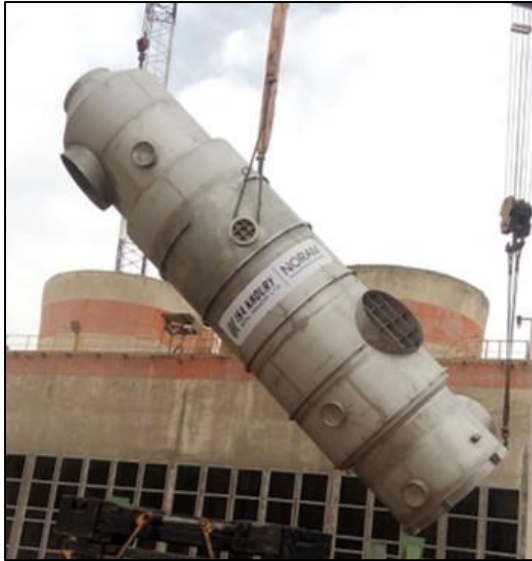
NORAM Gas Exchanger with Hot Sweep Installation
