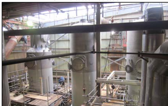
NORAM Dry, Interpass and Final Absorption Towers
