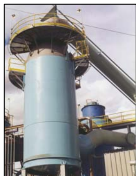
NORAM Acid Tower
