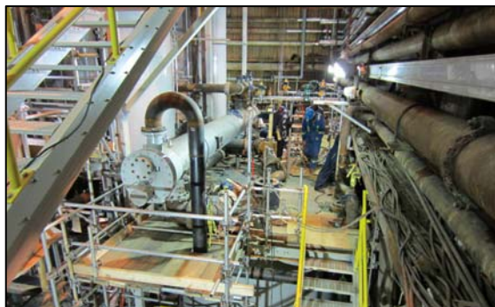
NORAM Circulation Acid Cooler
