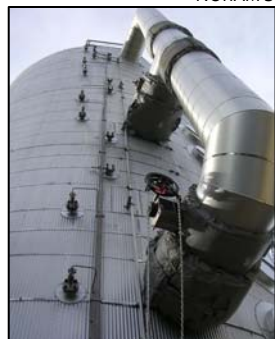
Converter Preheat Ducting
