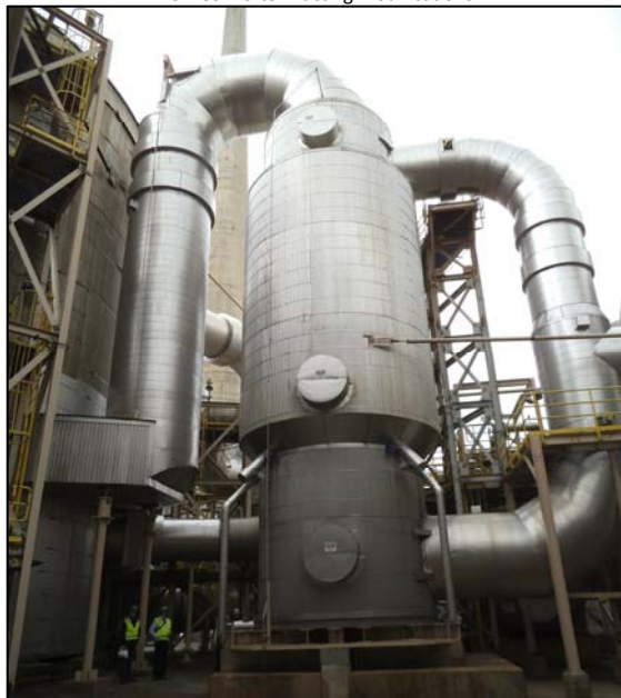
NORAM Cold Interpass Heat Exchanger
