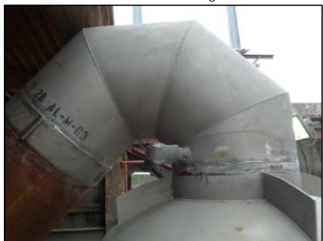
Absorption Tower Outlet Ducting
