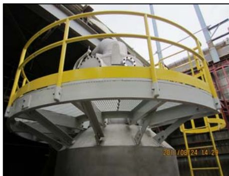
Absorption Tower Platform
