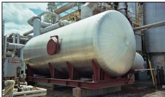
NORAM Sulphur Furnace
