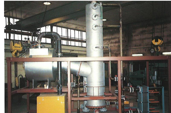
Skid-Mounted CF Burner with Quench Tower
