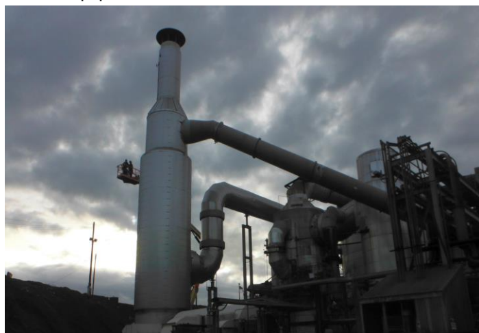
NORAM Preheat System
