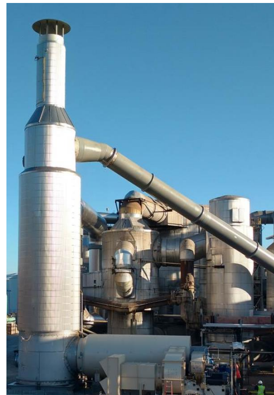
NORAM Preheat System
